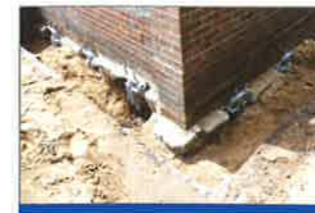
Overcoming Foundation Settlement
