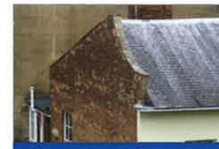
Restraining Bowed or Disconnected External Walls
